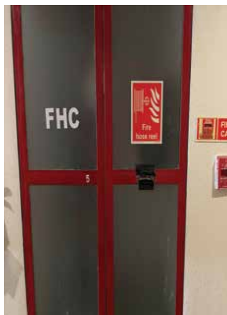
Internal fire hydrant system – Active fire
