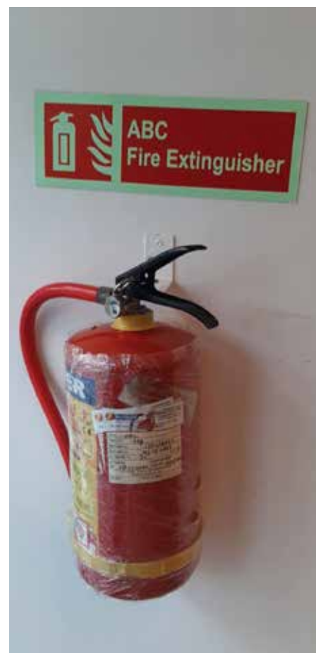
Fire Extinguishers – First aid appliance
