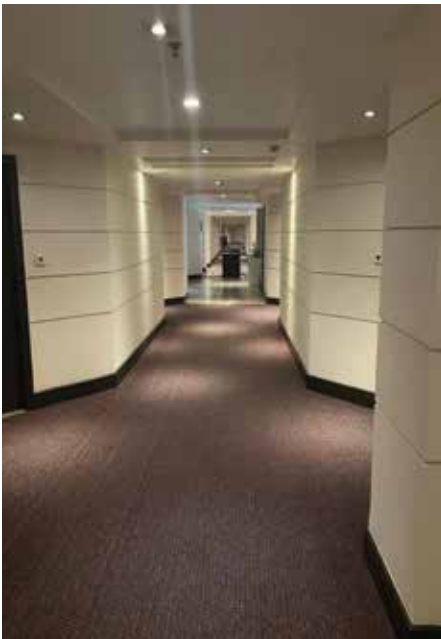
Escape route lighting
