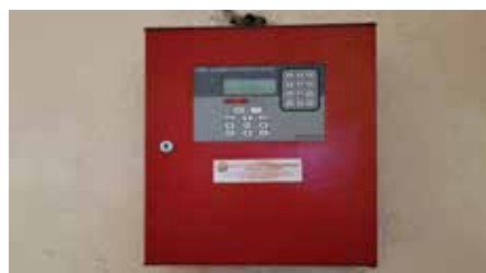
Fire alarm Panel
