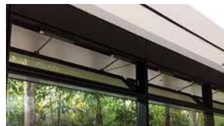
Automatic Smoke Ventilation Systems
