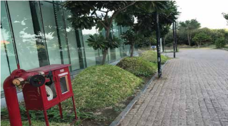
External fire hydrant system – Active fire
