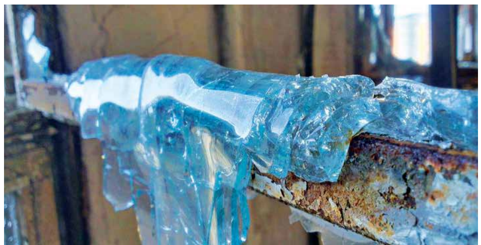
Glass melting from the window frame of a fire-damaged building
