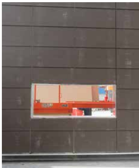
Picture 5: Contractors leaving the joints open without a filler
