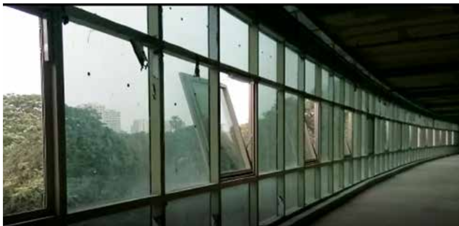
Automatic Smoke Ventilation Systems
