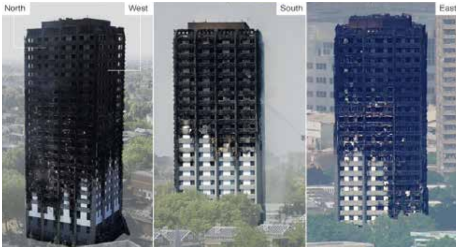
Grenfell Tower – Damage post-fire
